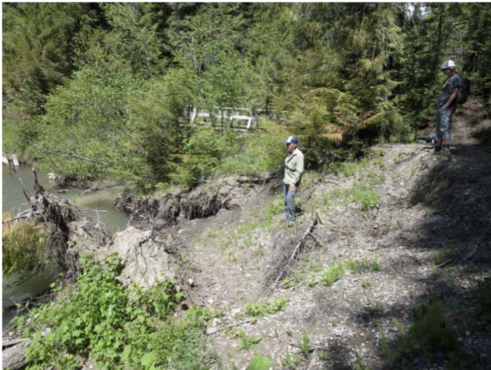
Figure 6 - Photo of Site 2 Slope Failure, July 2014
